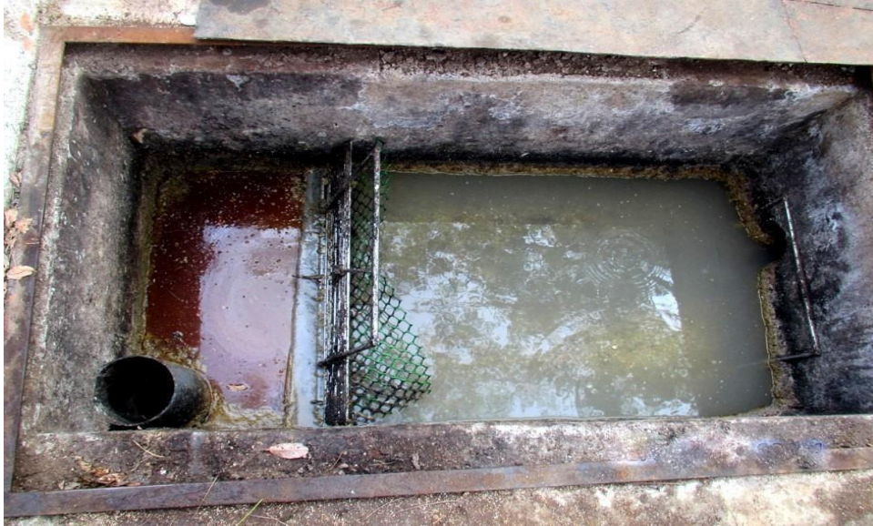
Figure 1.6 Tank for removing sediments and floating matter from canteen waste water before reaching ETP
